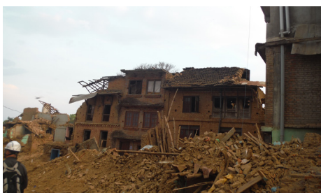
Traditional Newari houses constructed with brick and mud mortar in Dharmasthali, Kathmandu.
